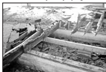
Damaged Lewis Grange hall floor.
